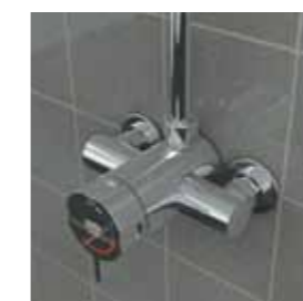
Exposed valve - top outlet
